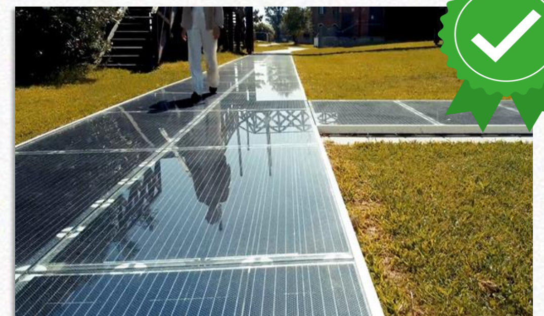
Cycle-pedestrian path PV system in Venice
