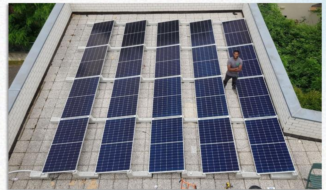
Photovoltaic system in Bologna
