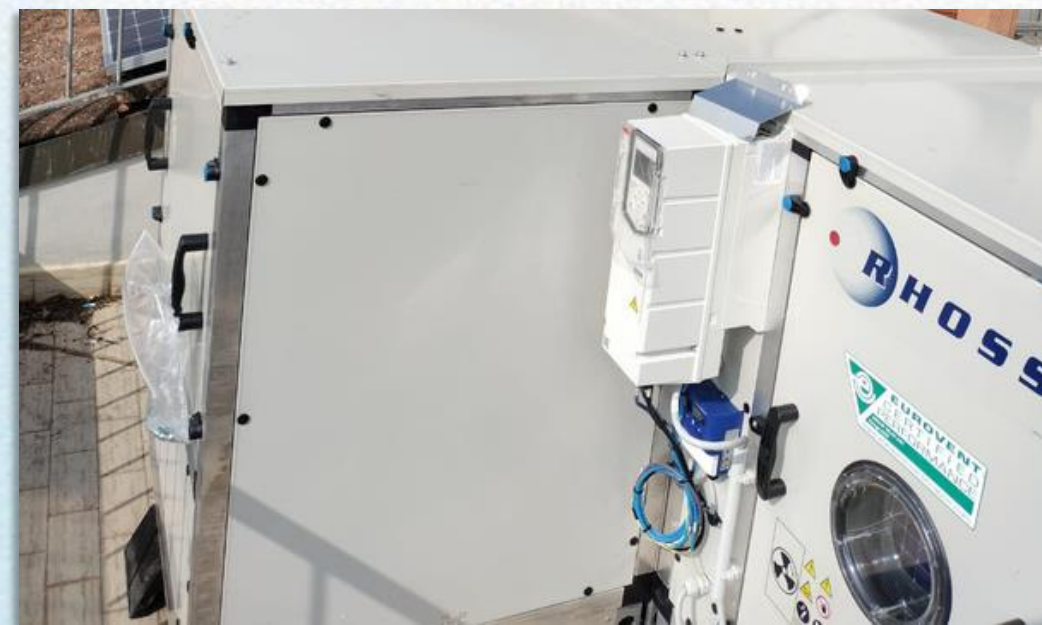
Heat pump in Ravenna
